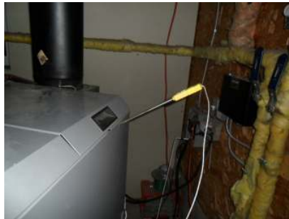
“K” type thermocouple measuring chimney smoke temperatures
