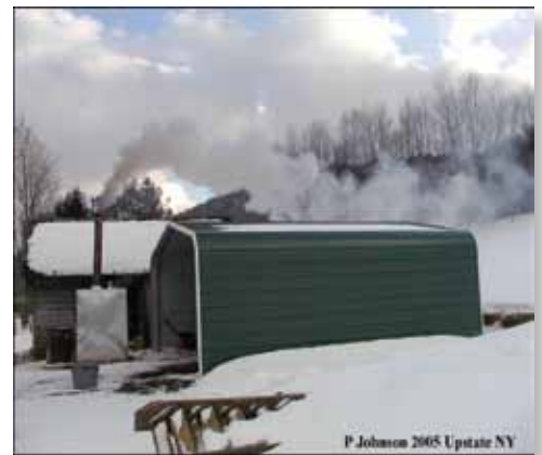
Outdoor wood boiler in Upstate New York
