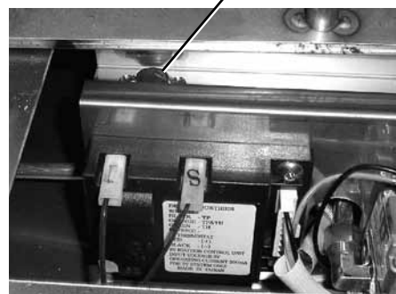
Limit Switch Location
